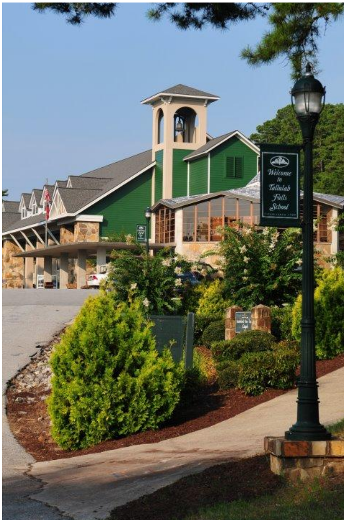
The new library has been completed at the school. The old library, pictured, will be gutted in preparation of its conversion into the new school entrance/lobby.
